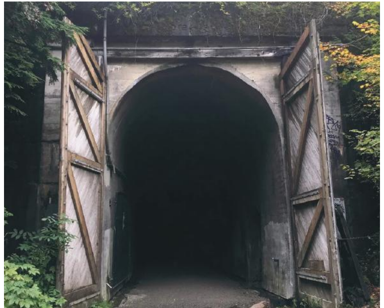
A photo of an entrance to the Snoqualmie Tunnel from during Mike Cyger's run from Seattle to Spokane. Contributed Photo / Mike Cyger
